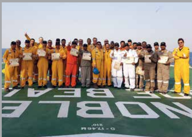
The Keppel FELS and Noble teams celebrating the successful repair of the leg of the jackup rig, Noble Joe Beall
